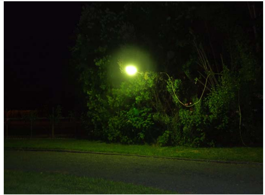
Old luminaire (96w)
